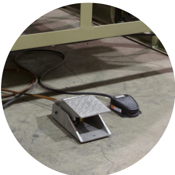
Blast and Turntable Controls
